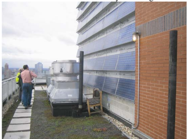
These solar panels would produce much more electricity if they were angled toward the sun, and were not shaded by rooftop equipment. As installed, they represent a colossal waste of perfectly good solar panels.
